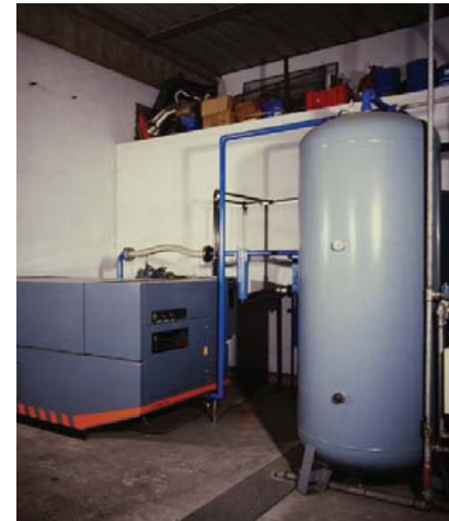
Figure 1-9. Pneumatic systems can easily store large volumes of compressed air to meet the intermittent high demand of some systems. The vertical tank on the right serves as a storage area for compressed air. (Photo: Atlas Copco)
