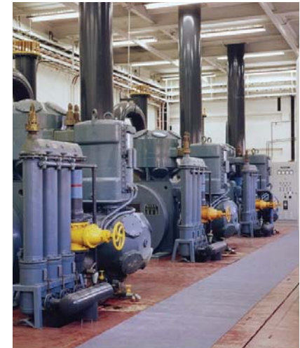
Figure 1-20. Central power systems are often used in large manufacturing facilities to produce compressed air for pneumatic applications. (Photo: Atlas Copco)
