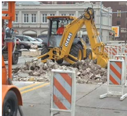
Figure 1-1. Equipment used in construction and street maintenance is an example of a fluid power application commonly encountered in daily life. This backhoe is capable of producing the brute force needed to break and move concrete. (Deere & Company)
